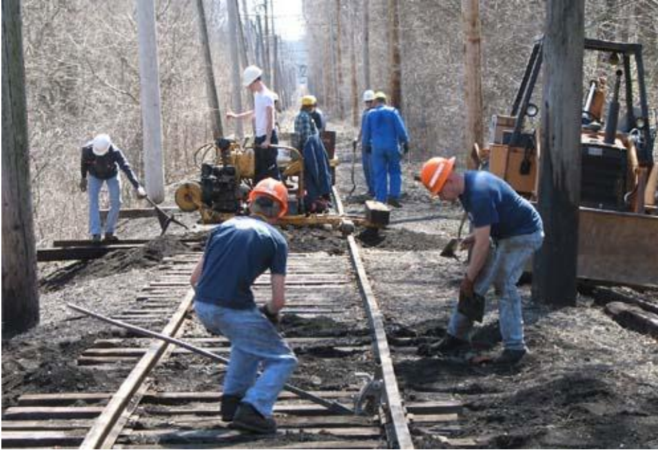
Adam Robillard and Frank DeVries plating ties in foreground, Chris Nelson and Matt DelGuidice using the tie inserter, and the rest of the crew ( Ed Konecki, Al Barker, Patrick Storm, Bill and Jim Minerly, and Chuck Galitz ) cleaning out slots for new ties.
