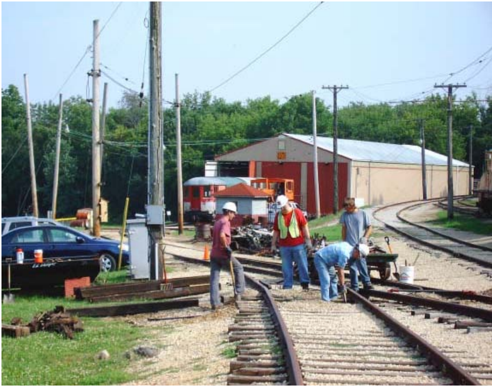
It was a bigger job than usual . . . replacing switch ties at switch 33N . . . They are bigger and heavier.
