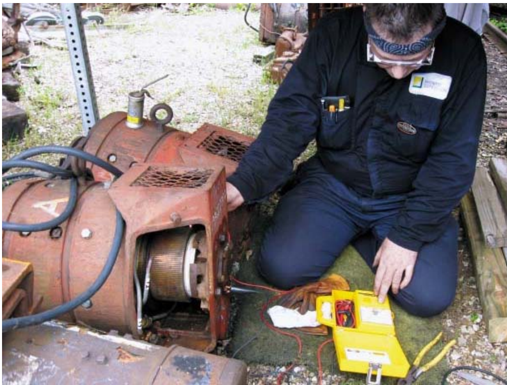
Chuck Galitz checking voltage potential on the "A" motor. Joe Hazinski
