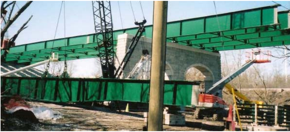
Large beams being readied for placement over the middle section of the bridge. Ed Tredup
