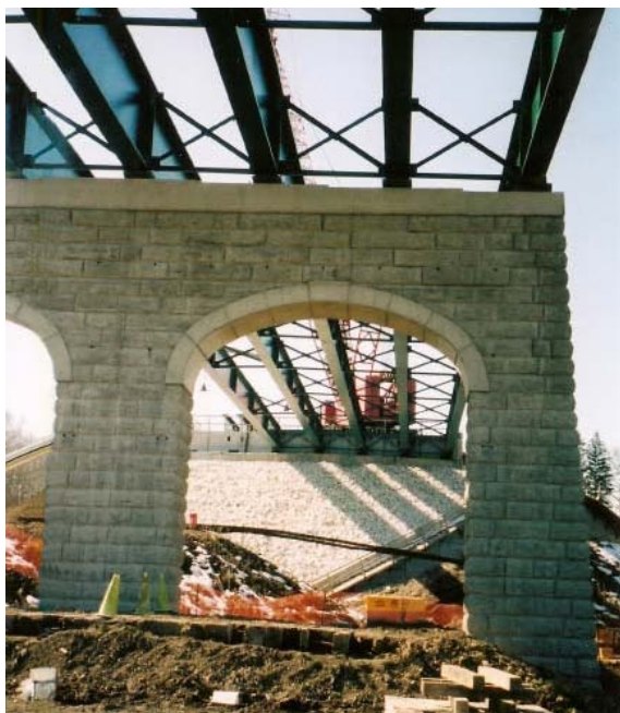
This spring shows beams in place as seen from underneath and awaiting the decking and concrete for the roadway. Note the special work in the concrete of the piers to give a "rock" appearance matching those of the CN's bridge. Ed Tredup
