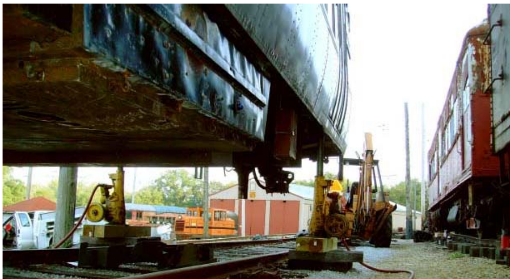
A worm's eye view of the underside of CTA #40 with the south truck removed. Note the jacks holding up the car while work is ongoing installing the refurbished motor. Don MacBean
