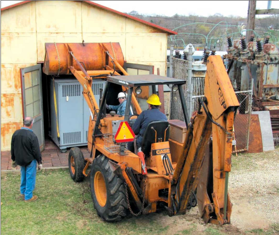
Left: With Chuck Galitz at the controls of the Case tractor a new transformer is guided into the sub station doorway by Bill Minerly as Jim Gonyo looks on in April 11 th , 2011. This transformer will better serve our 600 volt DC power needs.
