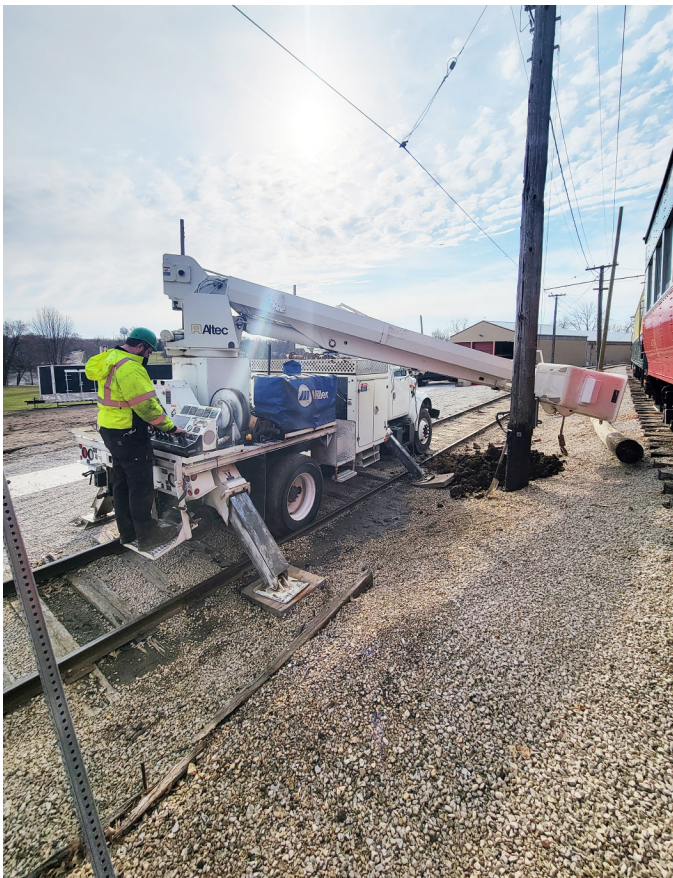
The line crew has picked a beautiful day to use the bucket truck to dig their holes
