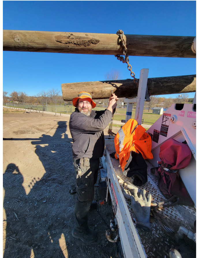
Jeff secures both poles to the truck after the team has picked them up. They will then dig two holes and place their poles.
